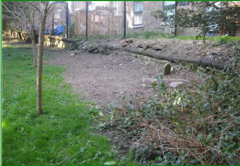
Note the damage and threat to the boundary wall now revealed
