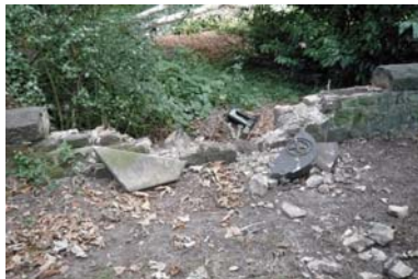
Parts of broken headstones and the damaged wall.
